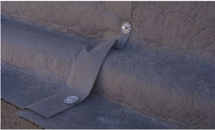
At the bottom, EnkaDrain is covering the pipe, no need of additional gravel material
