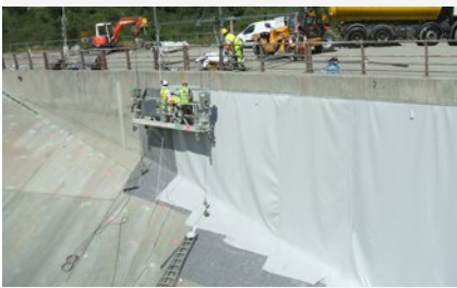
Use of a lifting platform to install EnkaDrain and PVC geomembrane on the diverter's abutment.
