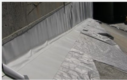
View of the diverter's abutment completed with vents and stainless steel flats fixed by screws
